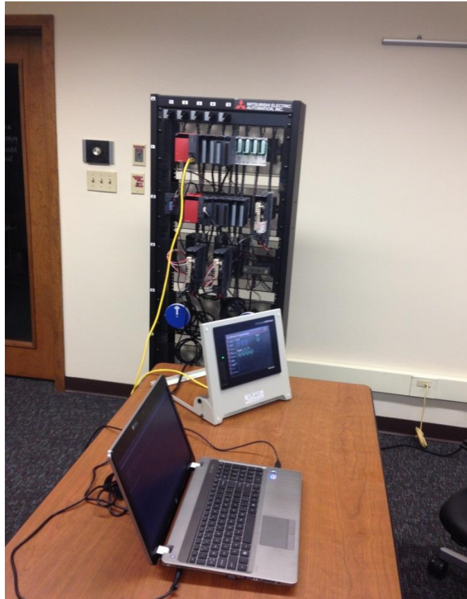
Figure-1 Trainer Rack with HMI and Computer
