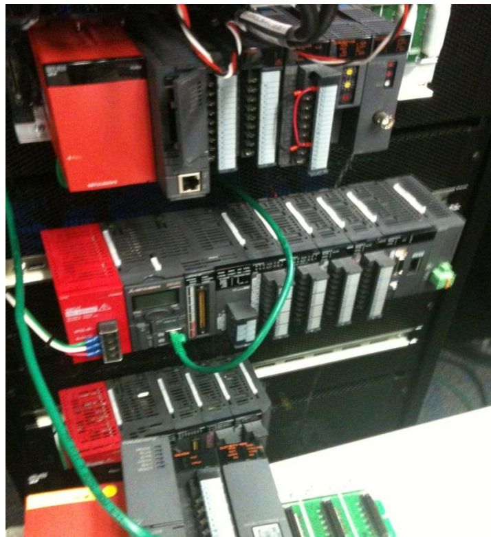
Figure-3 Tainer Rack with Different PLC modules
