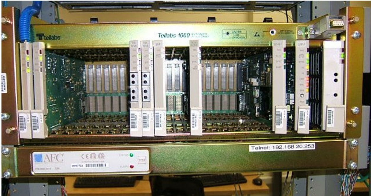
Figure 2 Optical Line Terminal
