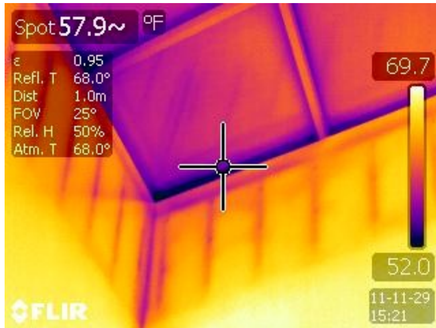
Figure 1: Thermal image of the interior wall and skylight of the atrium of the Business and Engineering Center. The cold studs in the walls are clearly visible in the image.
