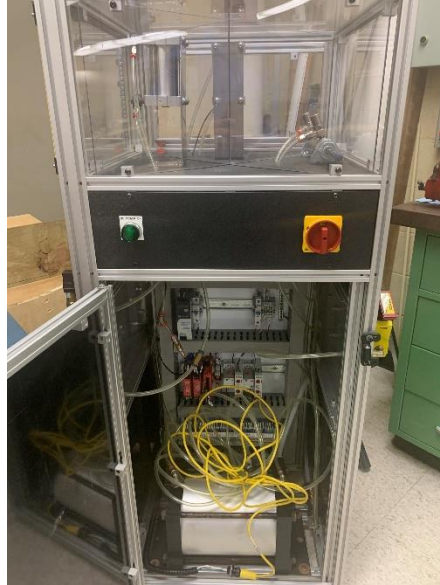
Fig. 10. PLC with integrated safety relays.
