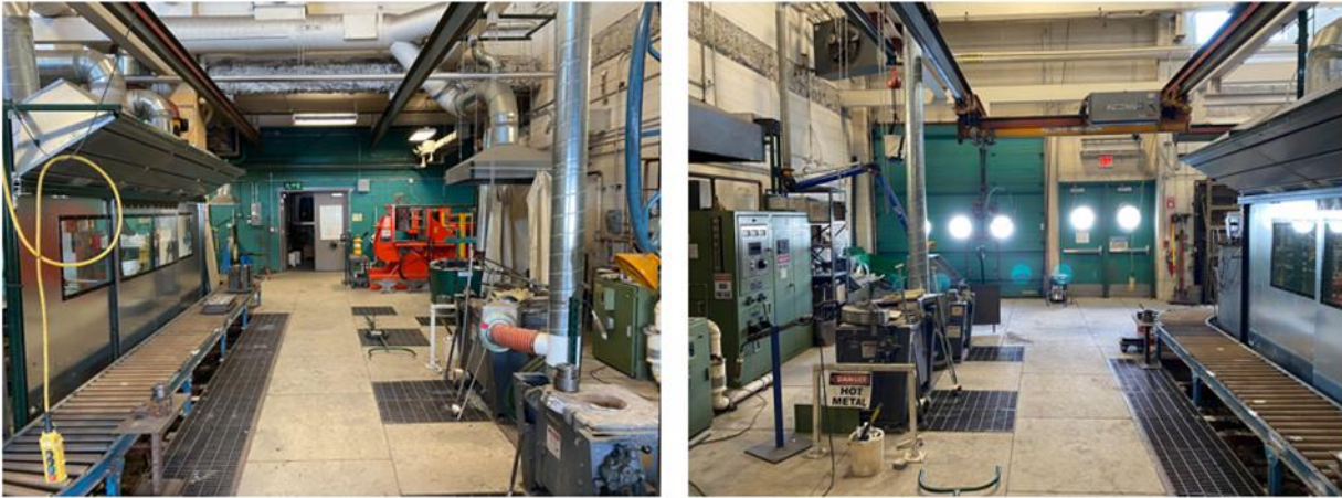
Fig. 4. Closed circuit cameras installed to track the casting process.
