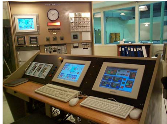
Fig. 2 View of reactor control room.
