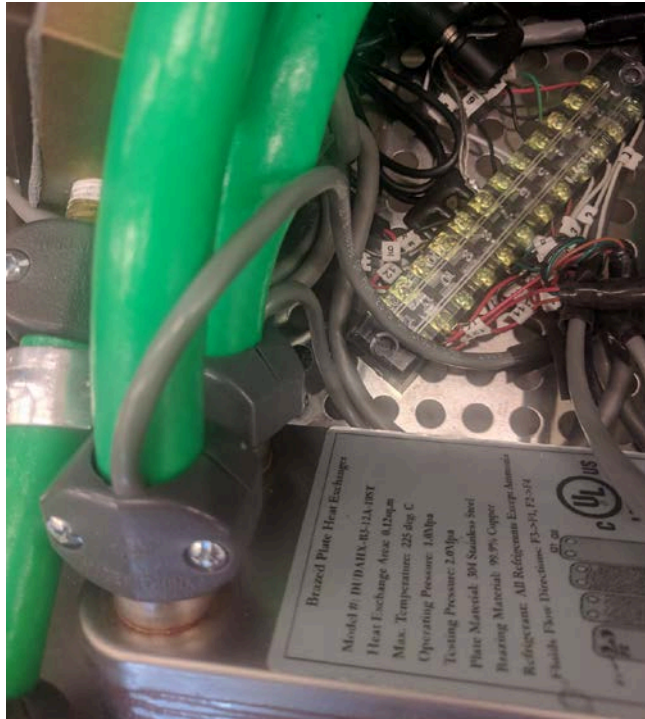
Figure 4. The electrical wiring of the heat exchanger test apparatus has been designed for easy identification and access for troubleshooting.
