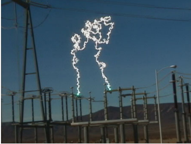
Figure 8: Photograph of a 500,000 Volt switching at Eldorado Substation in Boulder City, Nevada. Substation owned by Southern California Edison. 6
