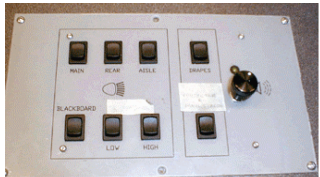
Figure 2. The HC-12 controlled physical button panel as an alternative to a graphical touch-screen interface. This panel provides manual override control of the room lights, projector, screen, drapes, and volume, without the need for distracting, hierarchical menus. Furthermore, the volume knob is context-sensitive, adjusting either the volume of the VCR when a tape is playing, otherwise, that of the instructor's microphone.
