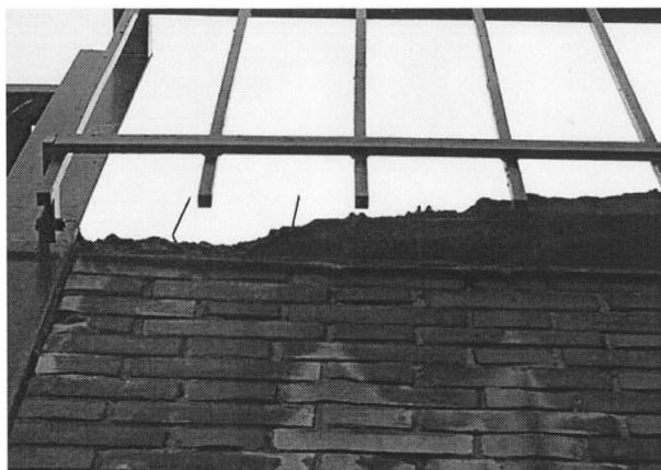
Fig. 4. Side view of deteriorated concrete deck. The concrete slab is intact on the right hand side, but on the left the concrete has eroded to almost full-depth.
