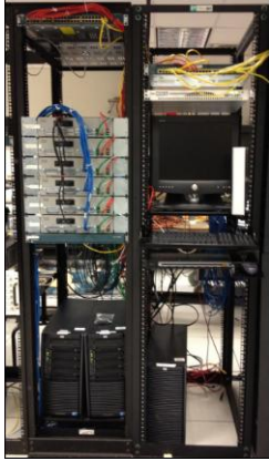
Figure 1. IPv6 Security lab equipment.
