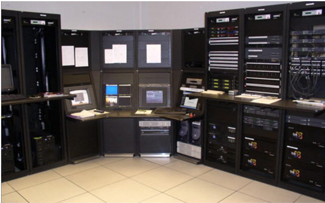
Figure 5. Global Classroom control room.
