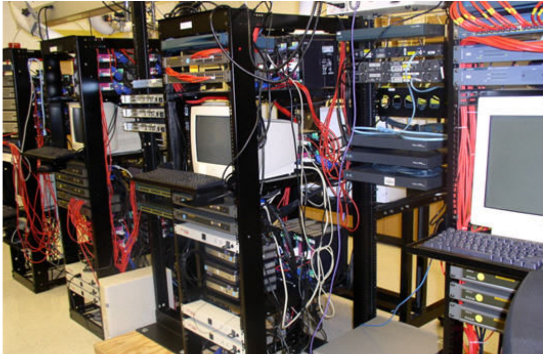
Figure 3. Operating systems and network management racks.
