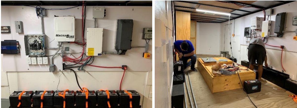
Figure 8. Actual electrical components installed on the panel board in the trailer based on the proposed design shown in Figure 4.
