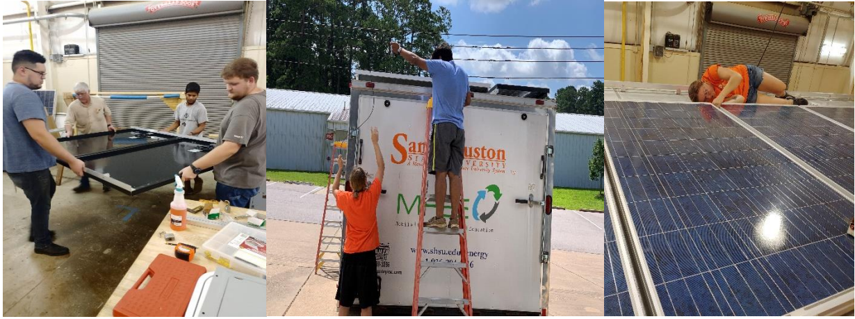
Figure 5. Student team members working in the MRRT project to precisely install PV frames and panels.
