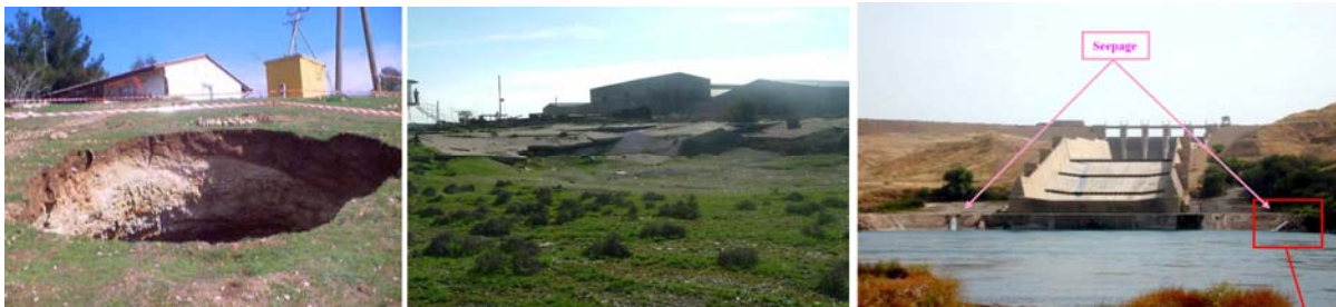
(a) Example sinkhole (b) Sinkhole beneath paved area (c) Example seepage
