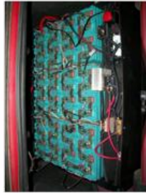
Figure 2: This photograph shows the 21 kW Li battery as it is mounted in the vehicle's trunk.
