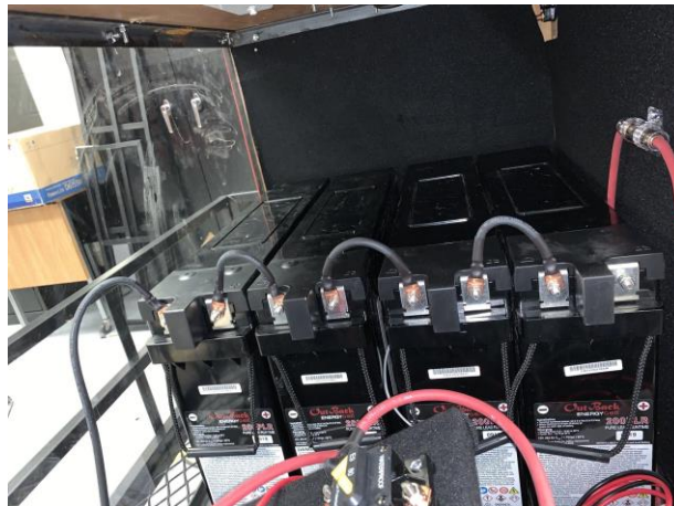
Figure 10: Batteries in storage box
