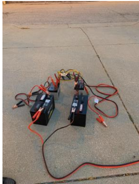
Figure 3: 12V batteries connected in series
