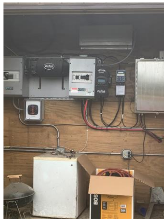
Figure 7: Horticulture off-grid combined solar/wind system
