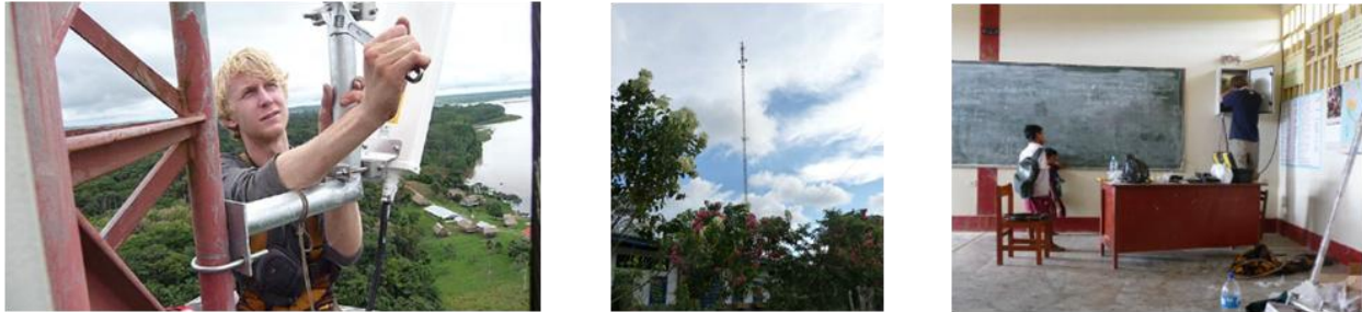
Figure 2: L-R (1) undergraduate researcher working on a tower; (2) network tower in Santa Clotilde; (3) undergraduate researcher installing a wireless router in the primary school in Campo Serio.
