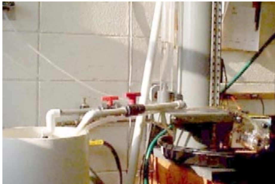
Figure 2. Photo of Level control station
