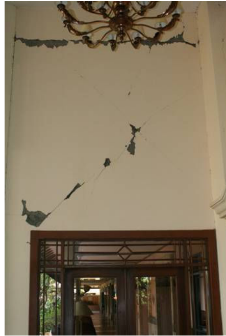
Figure 8: Assessing Earthquake Damage
