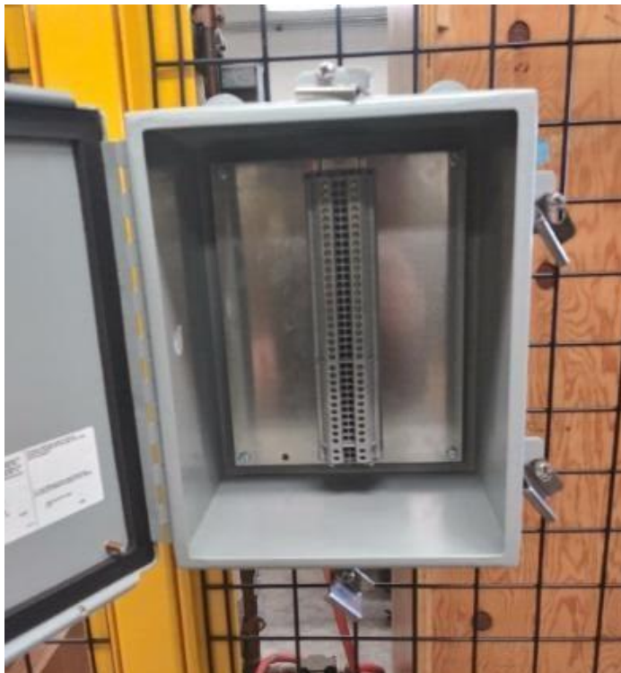
Fig. 7. The junction box and terminal block strip inside it meant for the 34 conductors from the cut cable coming from the controller cabinet.
