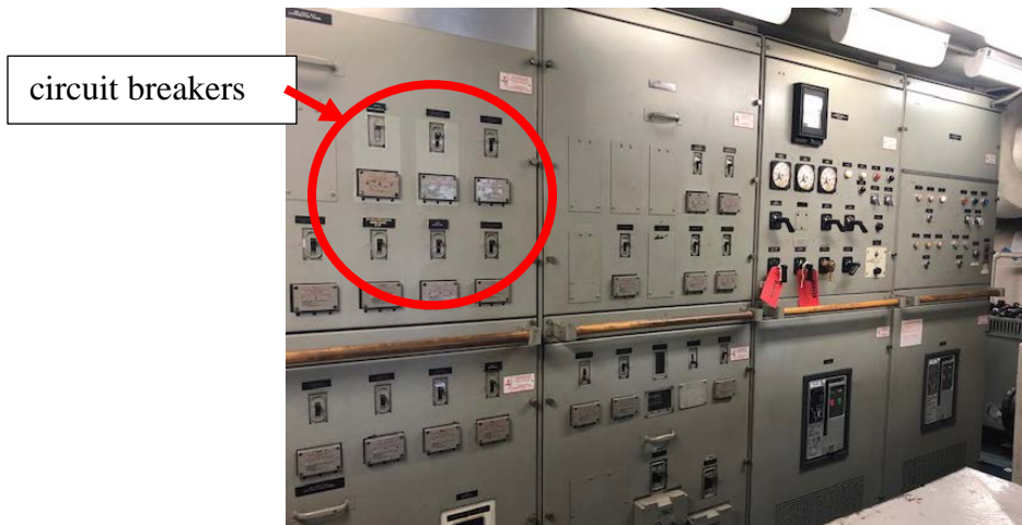
Figure 5. Ship's emergency switchboard
