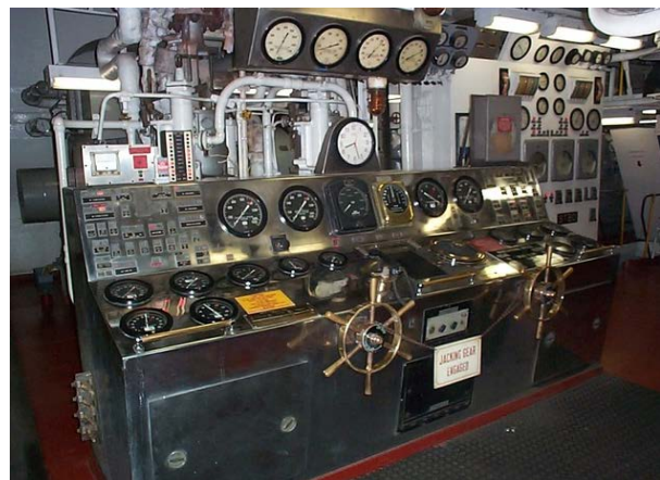
Figure 9. Typical steam plant control console
