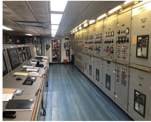
Figure 10. Diesel ship control console
