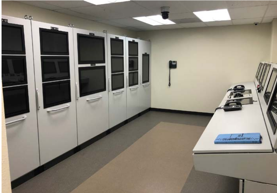
Figure 2. Diesel simulator I control room
