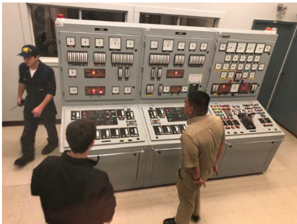
Figure 8. Steam plant simulator control room
