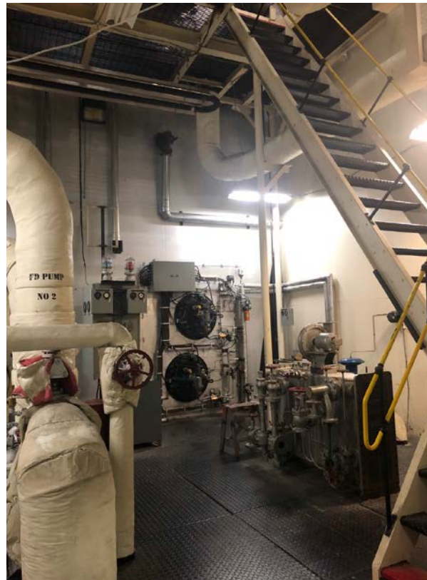
Figure 3. Steam full mission engine room
