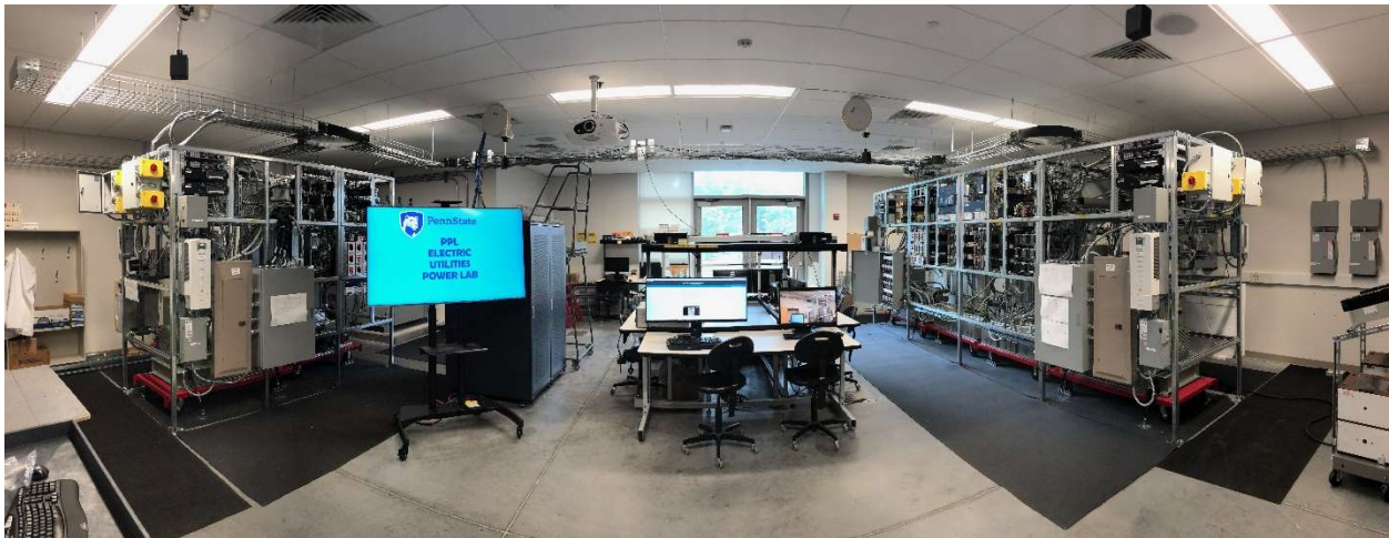
Figure 5. PPL Electric Utilities Power Lab – Microgrid Testbed.
