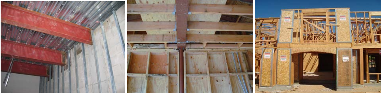
Figure 3: Interior View of (a) Steel Metal Deck, Steel Beams, Masonry Walls and Metal Studs, (b) Wood, Steel Girder and Steel Column and (c) Pre-manufactured Wood Shear Wall Construction
