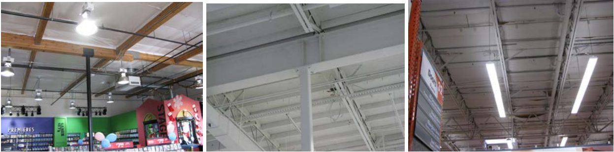
Figure 2: Interior View of (a) Glue-Laminated Beams and Steel, (b) Wood, Steel Trusses, Steel Girder and (c) Wood and Wood Truss Construction
