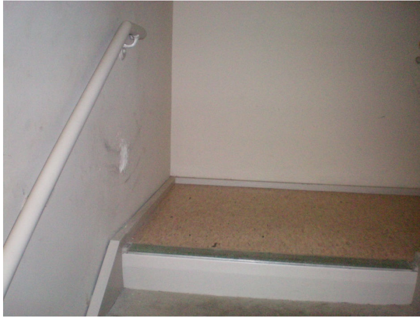
Picture 2: Paint peeling off an interior wall
