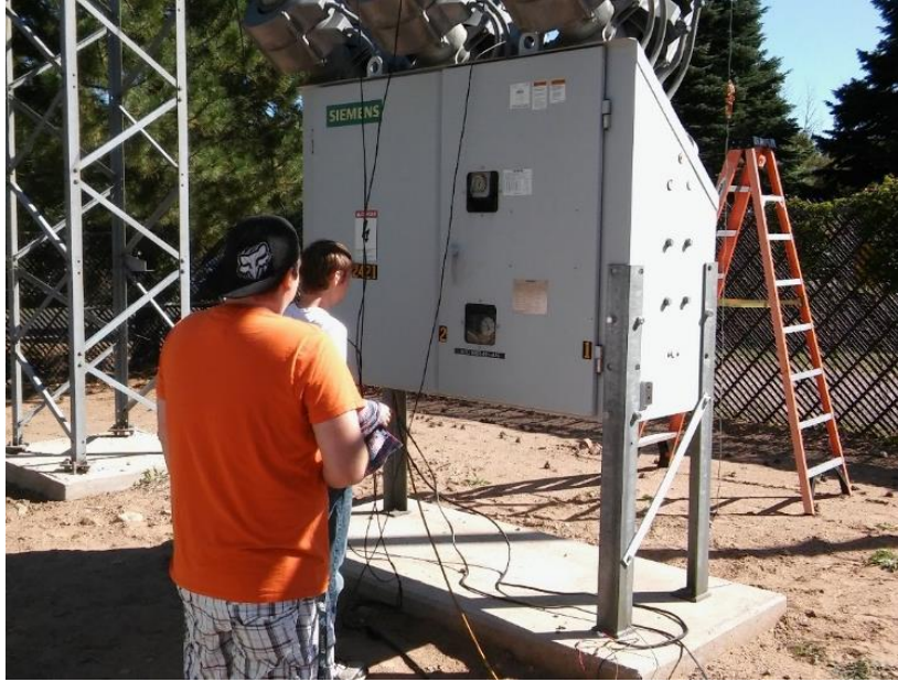
Figure 5. Students (Trayton Duncan and Kevin Wood) Observing the Circuit Breaker Travel Time Test
