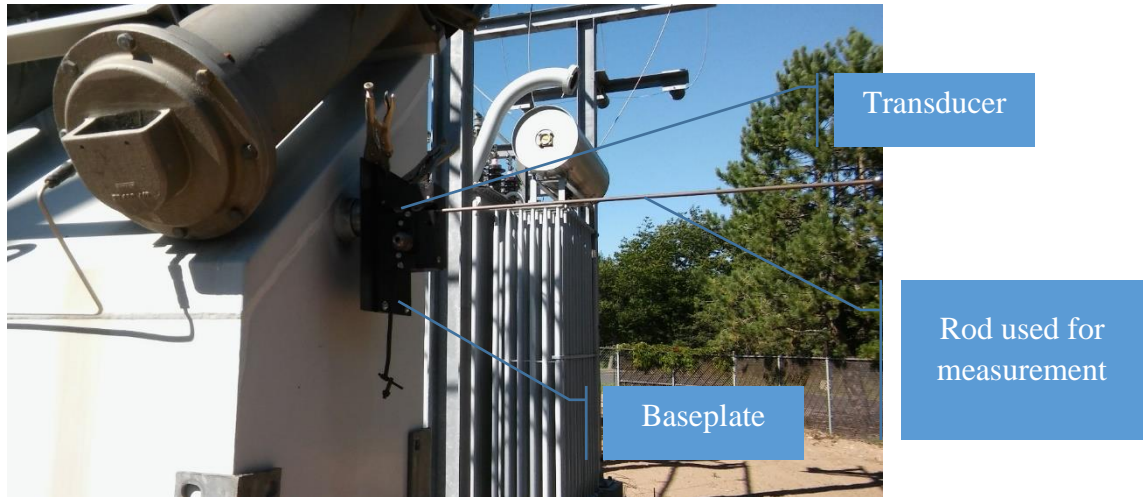
Figure 3. Displacement Transducer Mounted on Circuit Breaker with locking pliers and bolts
