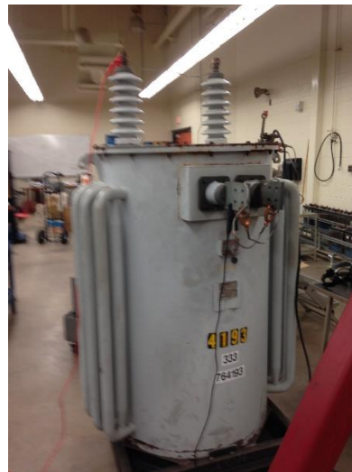
e. High-voltage winding to low-voltage winding
