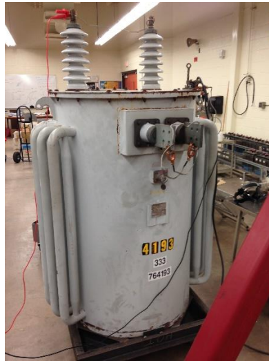
b. High-voltage winding to ground
