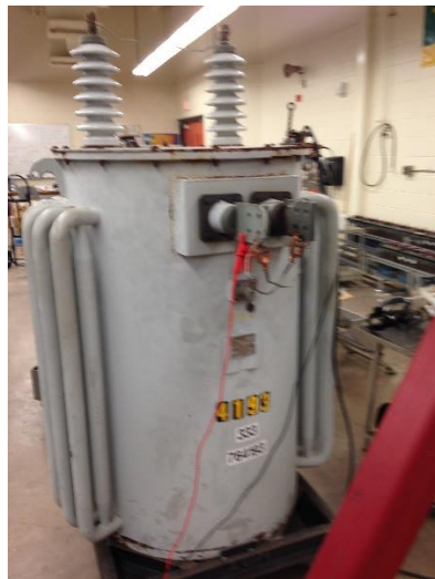
d. Low-voltage winding to ground
