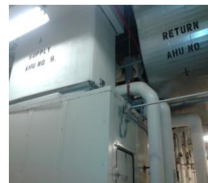
Fig. 7 The Pictorial View of Air Handling Unit (AHU)
