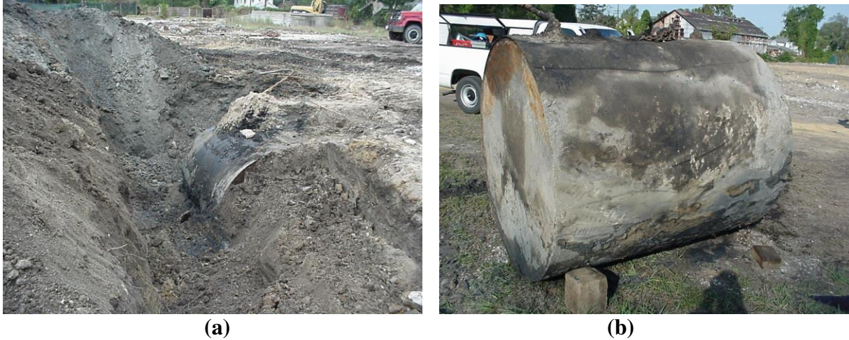
Figure 7 The Buried Heating Oil Tank
