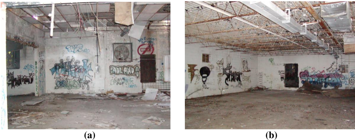
Figure 2 Graffiti on Walls, Rusted Steel Roof Trusses and Part of Collapsed Roof
