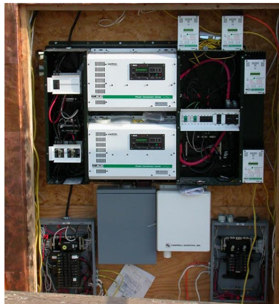
Figure 6: AC/DC Power equipment
