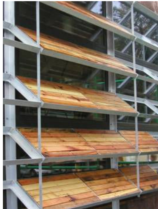
Figure 2: Louvers on the south side control the amount of sunlight entering the house.
