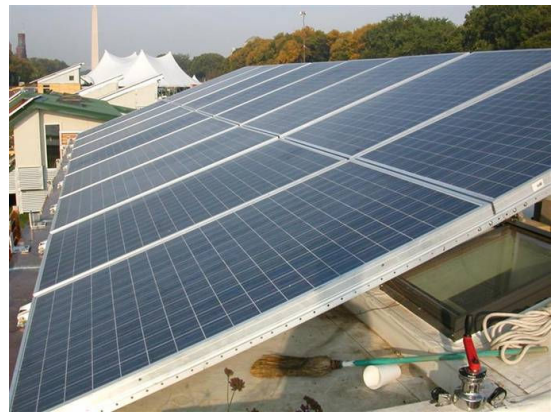
Figure 4: UVA Solar House photovoltaics.
