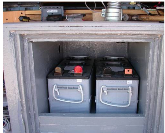
Figure 5: Two of the house's 16 batteries
