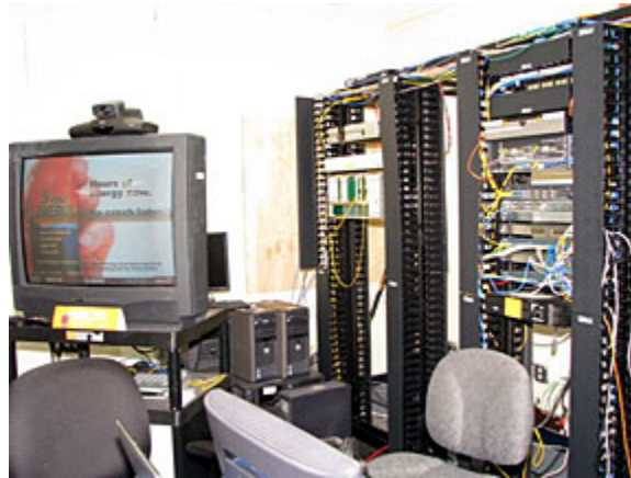
Fig. 2. Telecommunications Room 110-J
