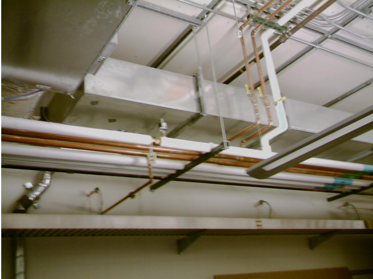
Figure 2.0, Portion of Instrumented Pipe.
