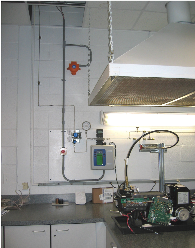
Figure 5: The in-laboratory hydrogen gas line that drops from the ceiling to the fuel cell test stand is illustrated. Pictured are the local hydrogen sensor, the orange disk on the wall in the upper center of the photo; the two-stage pressure regulator; one of the three the E-STOPS, located just to the lower left of the regulator; the pressure gage; the mass flow meter; the bleed valve and the gas line feeding into the fuel cell. The fuel cell is located at the lower right. A high – volume air ventilation hood used to vent any possible hydrogen gas leaks is located in the upper right of the photo.
