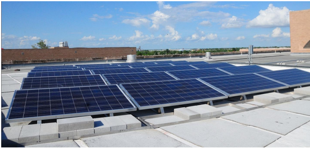
Figure 1 - ENGR PV Array
