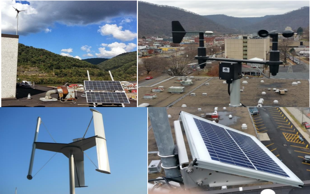
Figure 1: Residential wind turbines (both horizontal and vertical wind turbines), solar PV units, and weather station installed on the roof of the engineering building
