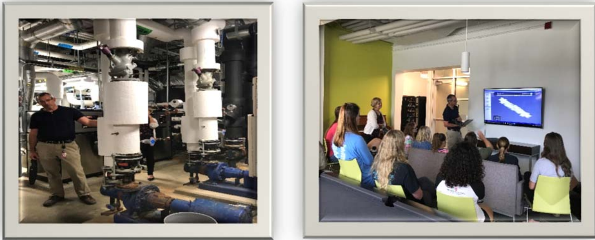
Figure 4: Photos from tour of Residence Hall Mechanical Room
