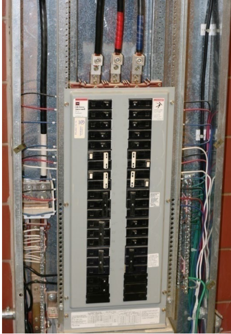
Figure 3: Example a building’s circuit breaker panel with the protective cover temporarily removed
